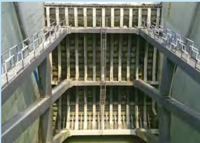
High Head (45 M) Top Seal Radial Gate erected at an elevation of 7216 ft., at Parbati Hydroelectric Project - Stage II (800 MW), Himachal Pradesh
