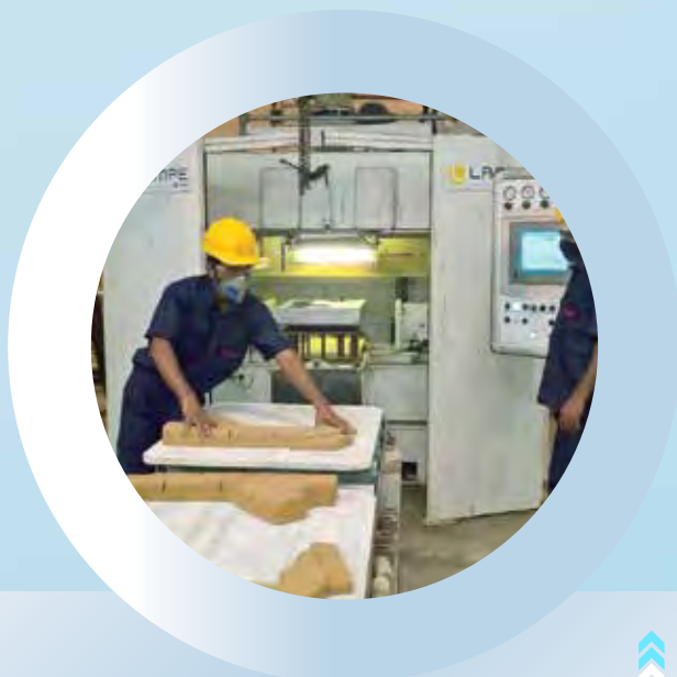
PLC controlled High Speed Core Shooter/ Blower from Laempe, Germany, installed at the Steel Foundry
