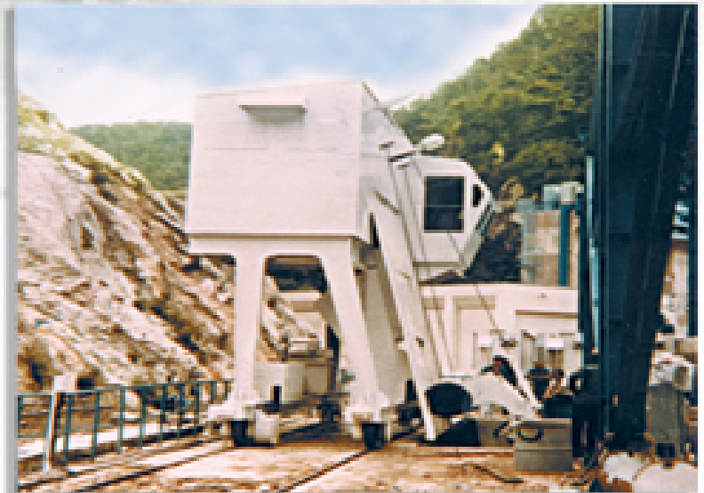
▲ Trash Raking Machine Tenom Pangli Power Project, Malaysia
