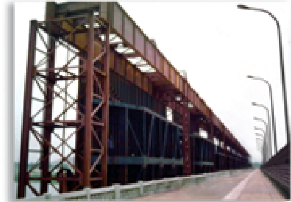
Vertical Lift Spillway Gates. Galudih Barrage, Jharkhand
