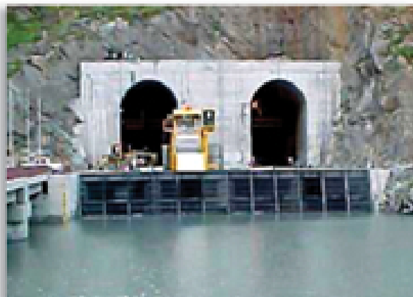
▲ Trash Rack Screen Chamera Stage-II, HP
